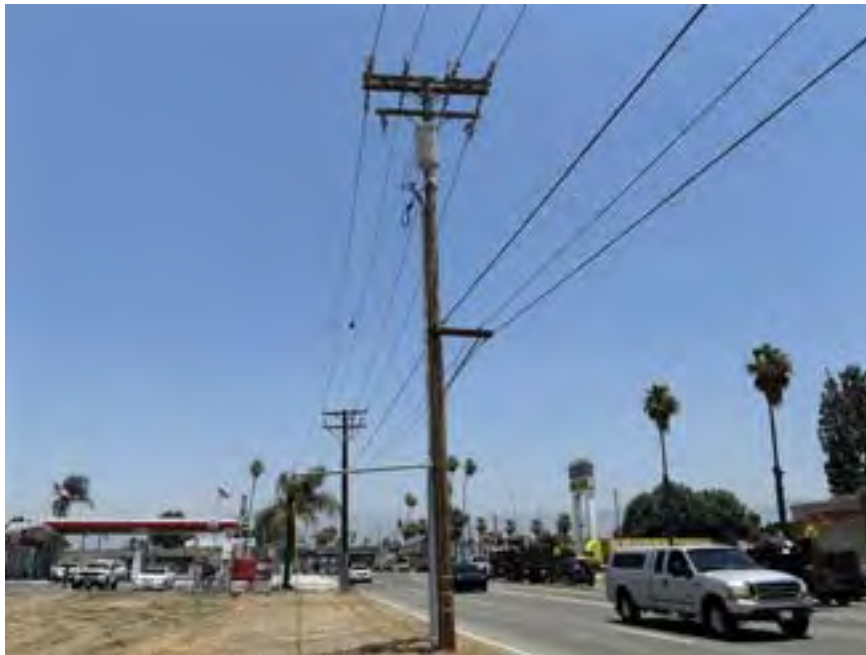
Photo 4: View of the pole-mounted transformer located adjacent to the north of the subject site. California Street is pictured to the right.
