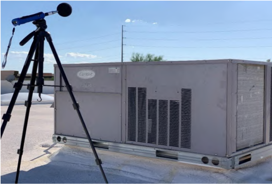
Figure 1: Commercial Air Conditioner - Carrier 50TFQ0006 - 5 Ton
