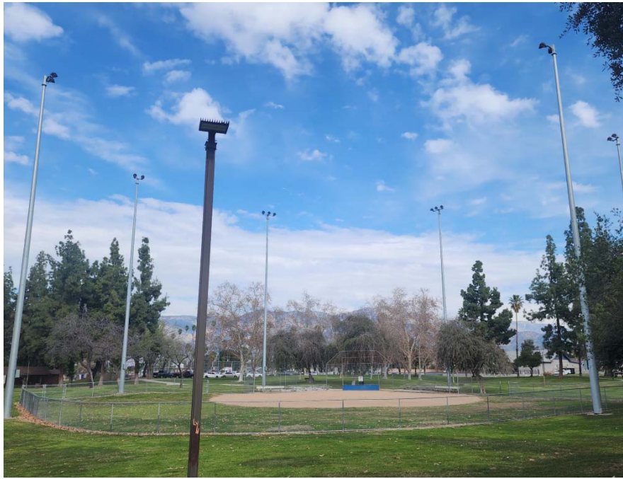
New Sports Field Lighting at Martinez Park
