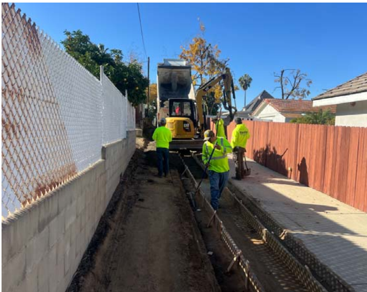
Setting Concrete Forms for the placement of the v-gutter in Alley from Division Street to Chapel Street.
