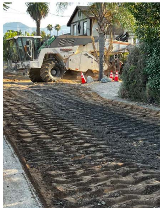
Grinding the existing pavement on Alley from Church Street to Division Street & Chapel Street
