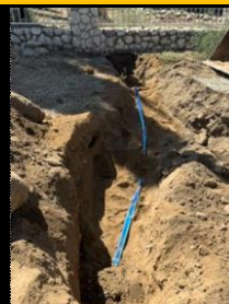
Water Service Lateral with Identification Tape on Mill Creek Rd
